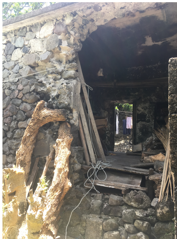
Figure 12. Examples of traditional homes in Itbud that were left dilapidated and abandoned. Many homes damaged by the 2000 earthquake, such as the bottom image used to be functional and liveable. Because DENR policies forbade the mining of lime for mortar and felling timber for construction, renovations and constructions were discontinued and the tradition of heritage house-building completely waned. June 8, 2019.
